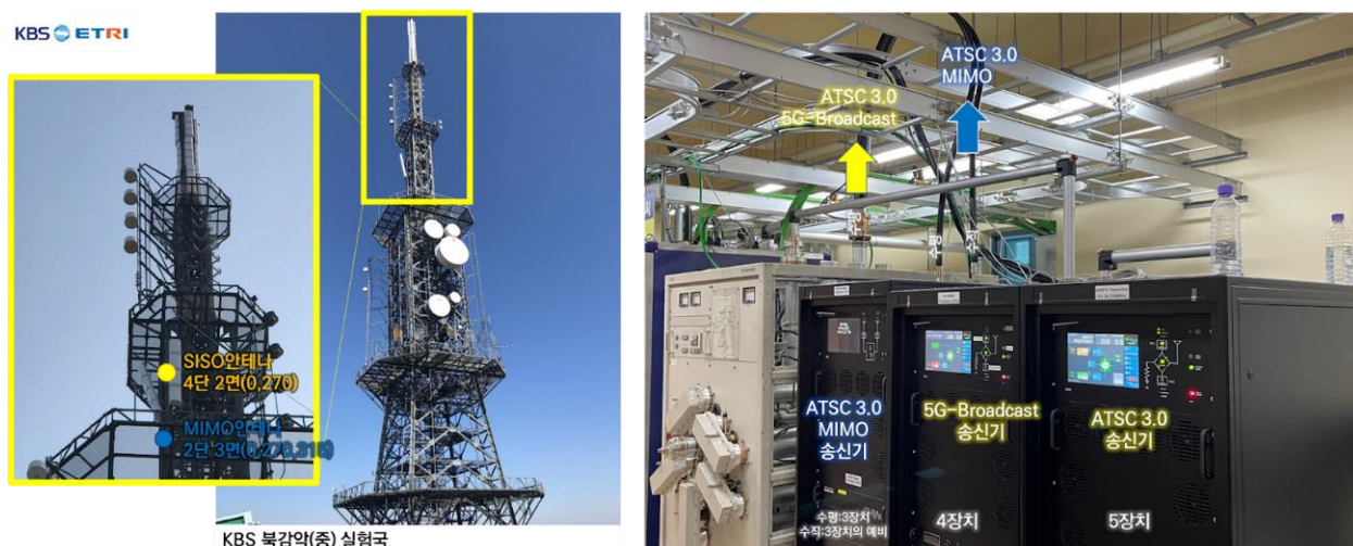
FIGURE 1.2.3 KBS Bukgamak Experimental Station (Left) 4-stacked 2-sided SISO antenna and 2-stacked 3-sided MIMO antenna installed on the transmission tower. (Right) Experimental transmitters installed in the 3rd-floor equipment room of the relay station. These devices have officially obtained South Korea's radio station permits.
