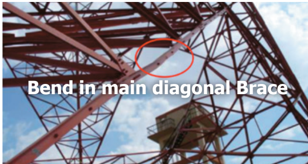
Figure 5: Bending in main diagonal braces
