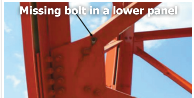
Figure 7: Fasteners missing in lower panel
