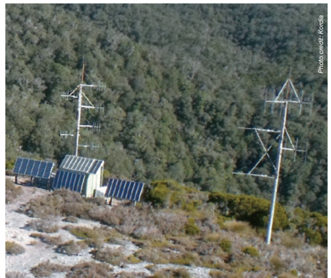
The Bald Hill analogue transmission site on the West Coast of the South Island, now closed. Its off-air input signal was from Paparoa, 230km away.
