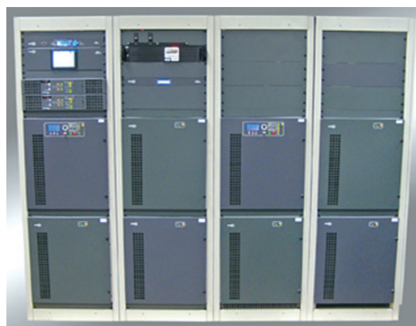
This is the actual 80 kW solid-state transmitter installed at this UHF broadcaster. It is now on the air.
